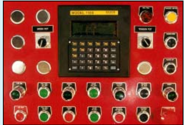
Main Control Panel
