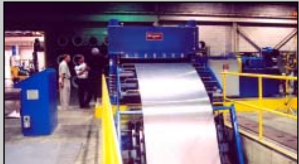
Hydraulic Leveler Producing Shape Corrected Strip
