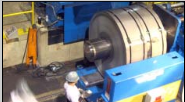
Slit coils unloaded by Floor Level Coil Car
