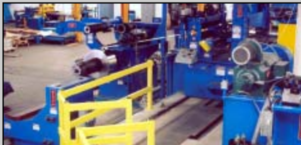
Double-Loop Slitting Line Entry End
